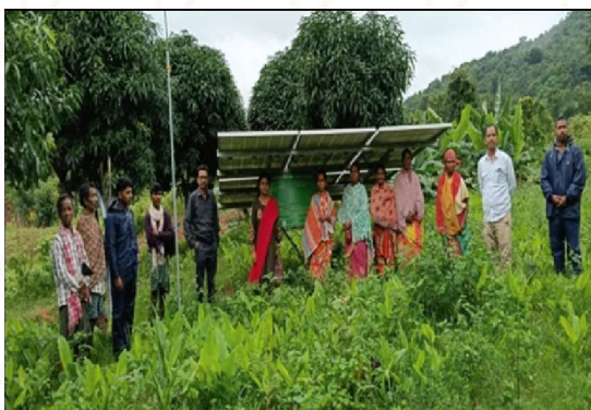
Solar borewell, Lanjigarh
